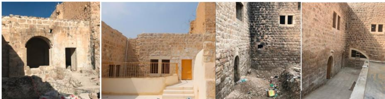
Figure No. (15) shows some maintenance and restoration works for Amr Palace. Source: Hebron Reconstruction Committee (2017-2018).
